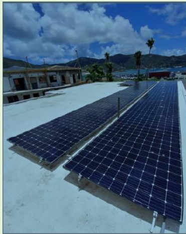
B: Solar panels on roof
